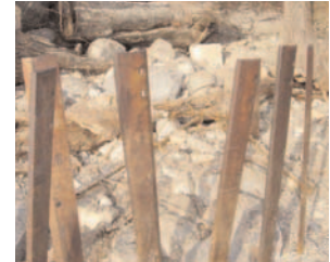
Failed barrier fence and rip-rap
